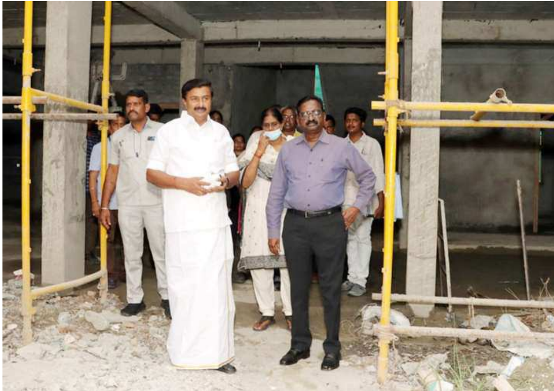
Hon'ble Minister for Tamil Development and Information along with Additional Chief Secretary to Government for Tourism, Culture and Religious Endowments Department inspected the new Administrative Building works on 30.06.2023, Government Museum, Egmore, Chennai
