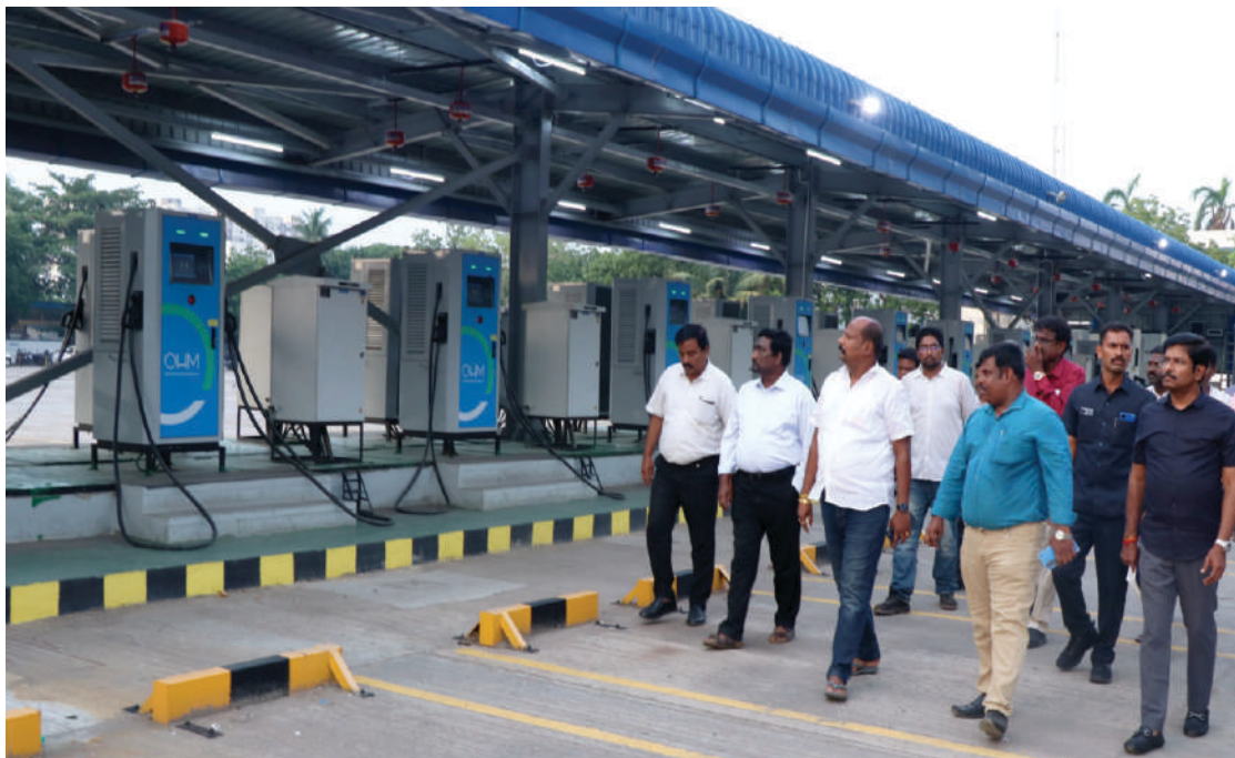
Hon'ble Minister for Transport, Thiru. A. Vijay Tamilan Parthiban, inspected the MTC Electric Bus Depot at Vyasarpadi on 11.07.2026 and reviewed the facilities and charging infrastructure.
