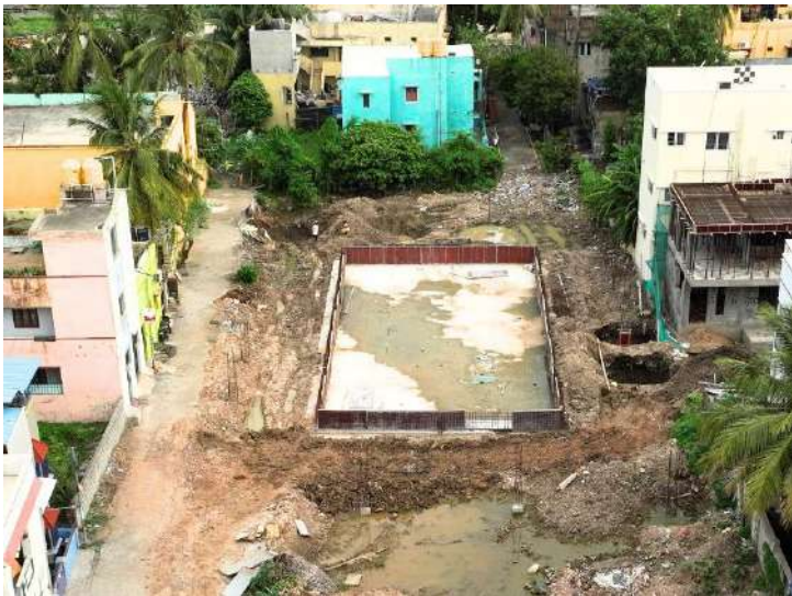
Construction of Chief Minister's Mini Stadium at Kolathur Assembly Constituency at a cost of Rs. 3 Crores
