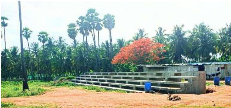
Construction of Chief Minister's Mini Stadium at Vaniyambadi Assembly Constituency at a cost of Rs. 3 Crores
