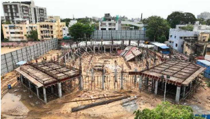
Progress of Construction at Gopalapuram Boxing Academy at a cost of Rs. 7.79 Crores
