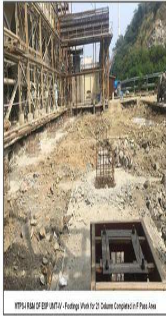
MTPS-I R&M of ESP Unit-IV: Erection of Inlet Duct and Gate for "F" Pass
