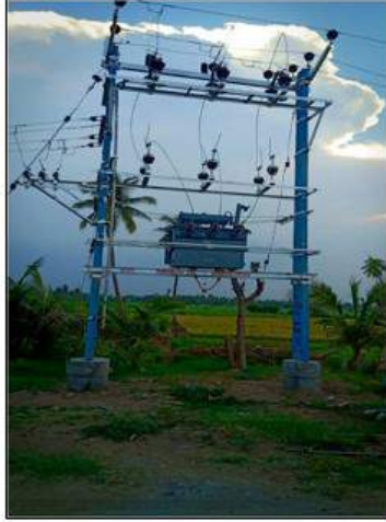
Nathamedu 22 KV Structure
